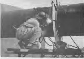
THE SECTIONS were carefully welded together. When completed, the line will be 8,000 feet long, and 3,600 pounds of welding rods will have been used.
